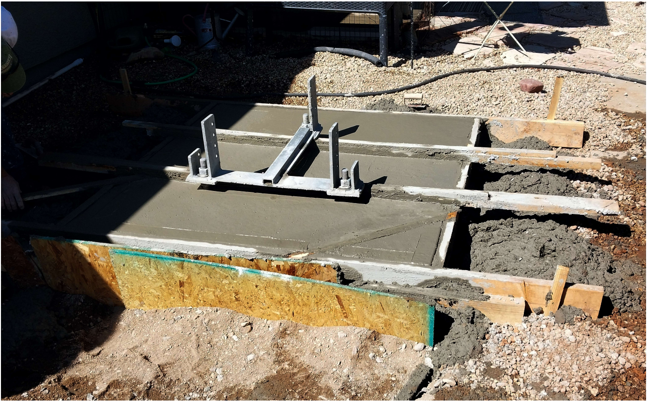
Poured cement for an antenna tower base at the home of Bud Winters N7BUD ▲ Prescott Valley, Arizona — April 12, 2025 (Photo courtesy of Bud Winters N7BUD)
