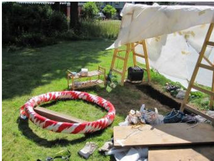
Loop ready for “grounding”. On the bench box and FM transmitter.
