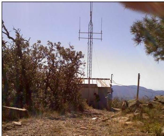
Jim (N6KZ) and Bud (N7CW) complete emergency backup power installation and testing at the Mount Union ARES/RACES repeater with Peter (W7PRG) (not shown), Lloyd (WA6ZZJ) (not shown) and Creighton (AD7YR) (not shown).
