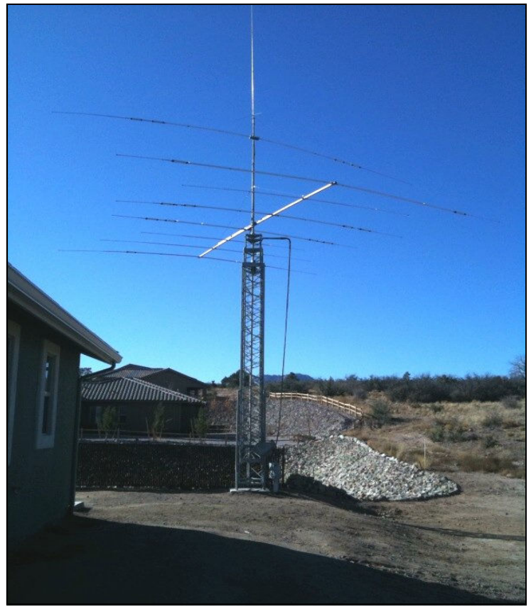
Final Antenna/Tower completed at N6KZ, Prescott, AZ
