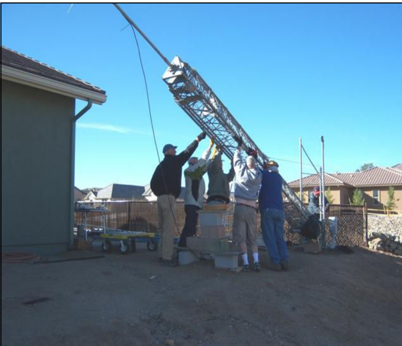
Tower being hoisted upright with hand-powered winch. Ground crew steadies tower and ensures smooth raising. Ray, N6VR, operates hand winch.
